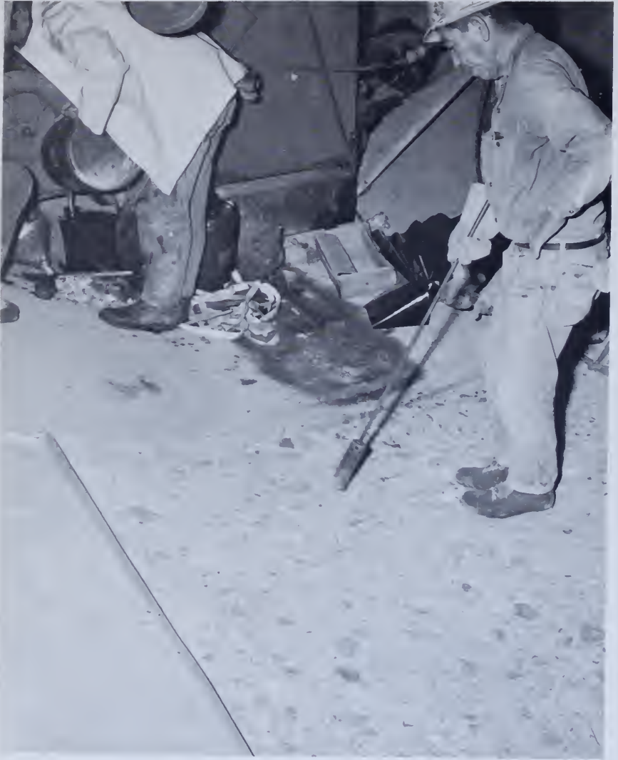
Figure 177. —A gas-fired weed burner being used to warm and dry an area prior to the placing of epoxy-bonded concrete in the spillway tunnel at Blue Mesa Dam, Colorado River Storage project. P622A-427-15030.
